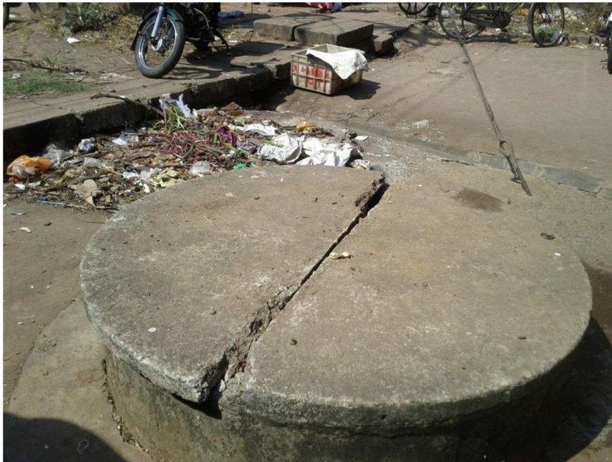
Tank made for waste water disposal but using as a waste dumping place.
